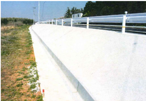
ฉ) Rode slope face sticking concrete
